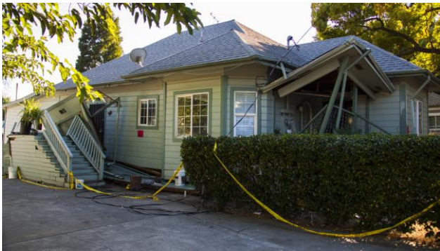
Napa, Calif., August 24, 2014 -- This house suffered severe damage after an earthquake shook up Napa, California. Building inspectors are going door to door assessing damage done to homes and businesses in the city to ensure that residents stay safe from falling debris and unstable structures.
