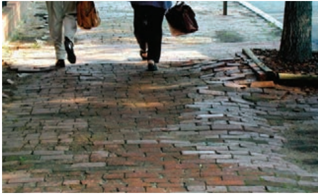
Pavers require regular maintenance to meet ADA requirements
