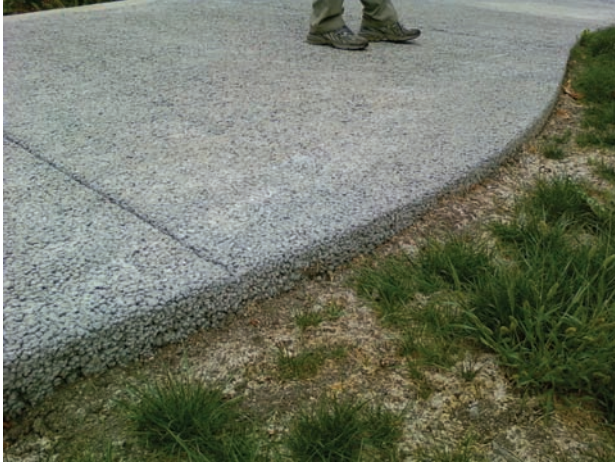
Concrete mix design is critical in pervious sidewalk to avoid a rough surface
