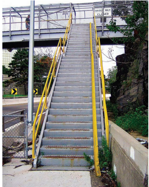
Metal channel (in yellow) provided for bicycle access
